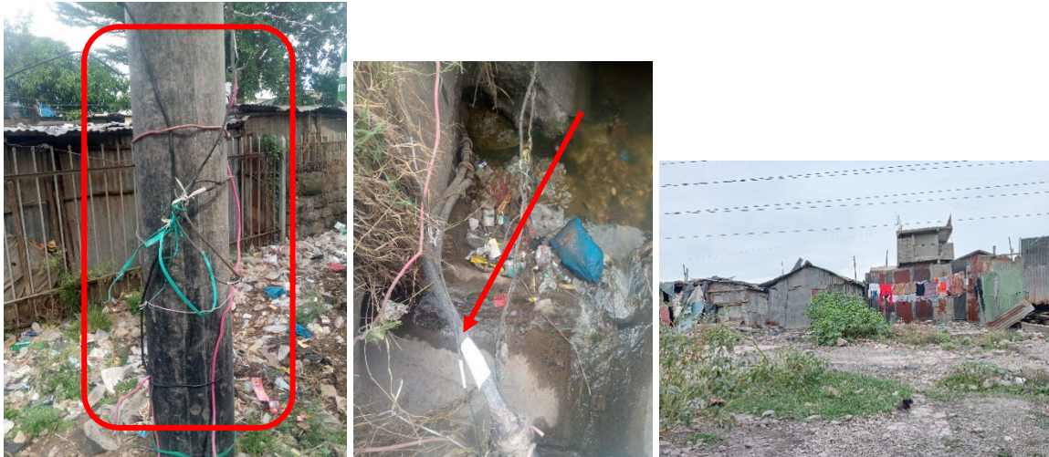
Photo 4: Left and middle: Cables used to tap electricity from nearby transformer, which is then used to supply electricity in the settlements. Right: Thin aluminium wires crisscrossing the settlements. Photo credits: Abigael Okoko
