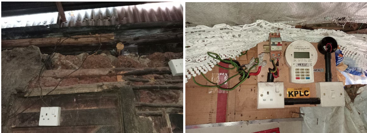
Photo 5: Left: Wiring in one of the households. Right: Vandalised KPLC token system in a household in the informal settlements
